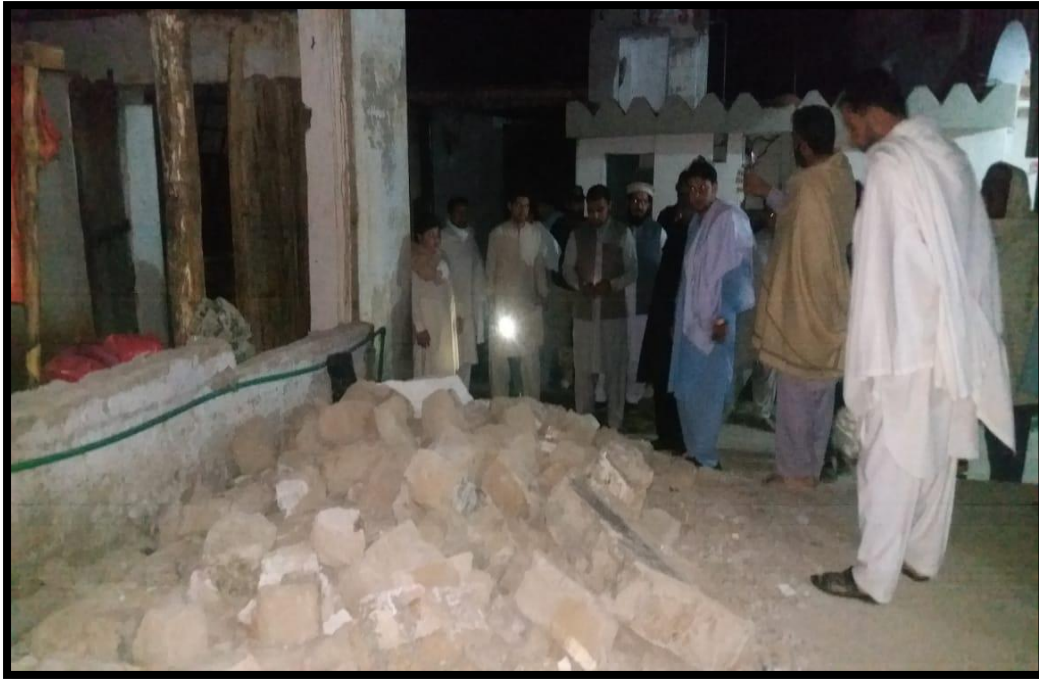
Roof Collapse in Swabi
